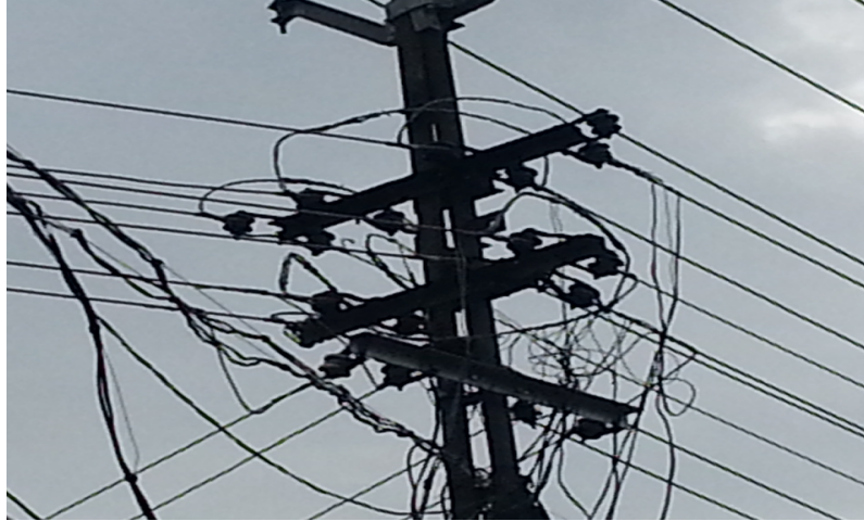
Figure 3.1: Non-technically managed low voltage distribution feeder
